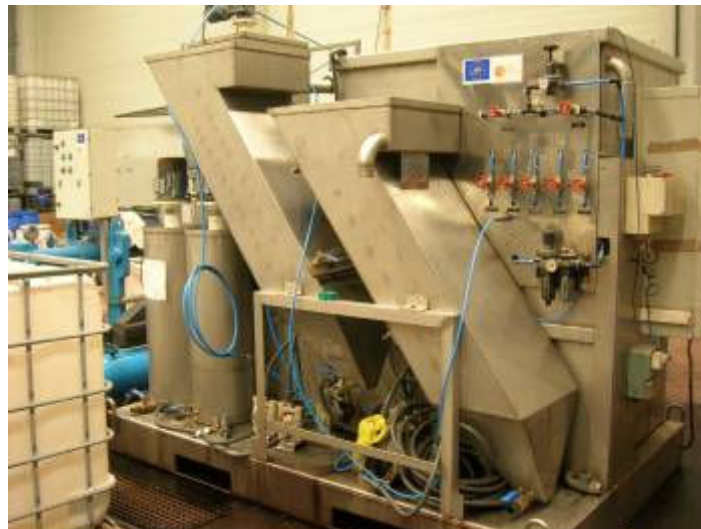
Waste water treatment plant
